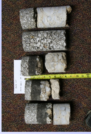
Road Coring Base failure forecasting
