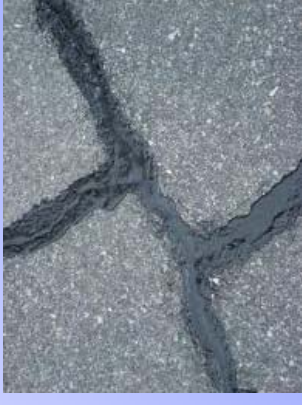
Crack seal 5 years post resurfacing
