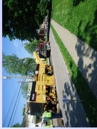
Base failure repair Determined prior to resurfacing
