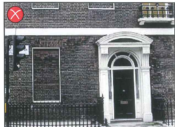
Bricked up openings are not permitted
