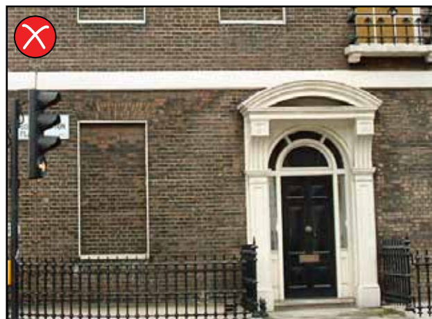
Bricked up openings are not permitted
