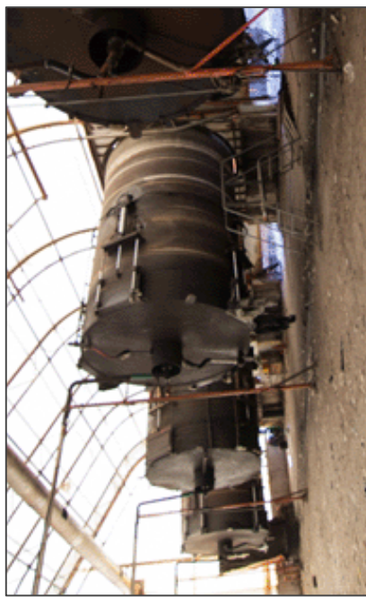
Sevierville Bio Digestion Facility
