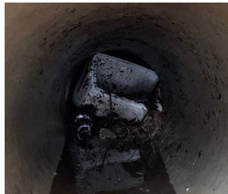
Coolers blocking Storm Pipes
