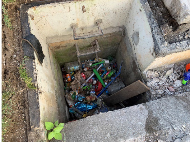
Curb Inlets full of Trash
