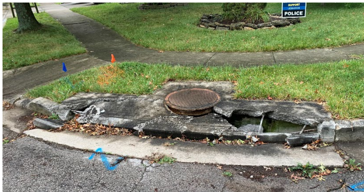
Completely Broken Inlets
