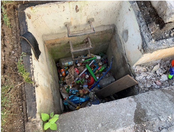
Curb Inlets full of Trash
