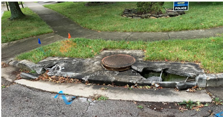
Completely Broken Inlets
