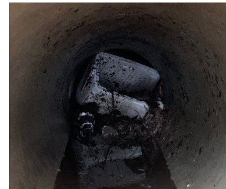
Coolers blocking Storm Pipes
